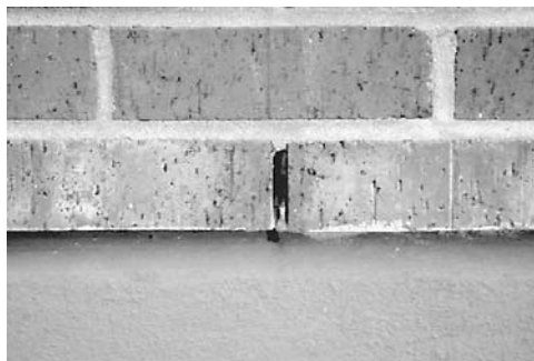
Figure 15-37 Mortar droppings can inhibit the drainage through weeps, causing efflorescence or other moisture damage.
